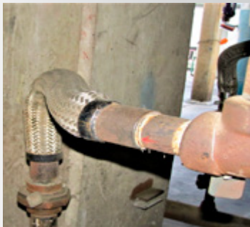
This metal braided hose has stressed and kinked behind the weld collar, due to inadequate routing.
