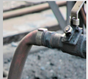
Air / water hose with only a single band, attached to a garden hose fitting, and kinked behind the band.
